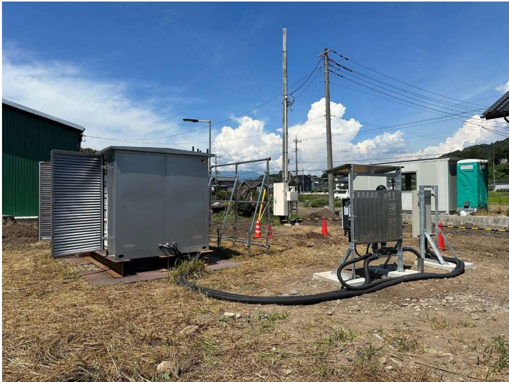
Containerized Data Center (Agile Energy X, TRIPLE-1)
