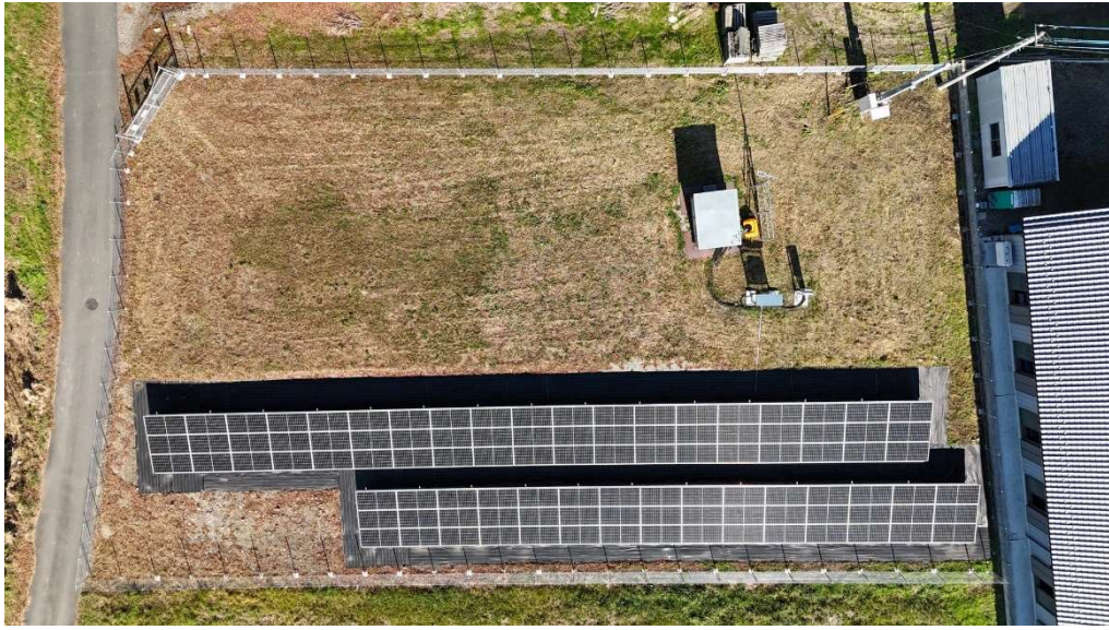
Solar Power Station (TEPCO RP)
